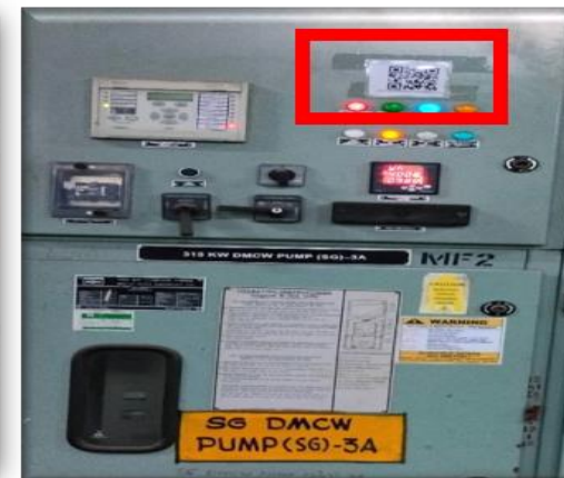
QR Codes scanners in Switchgears
