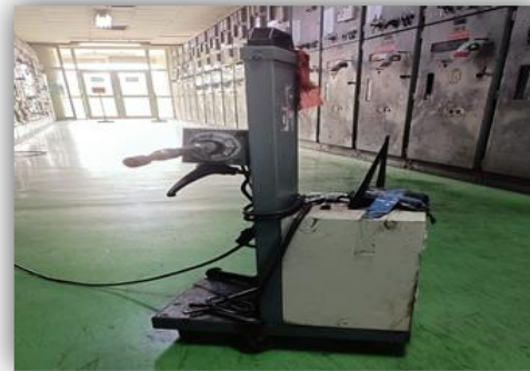
Remote Breaker Operation
